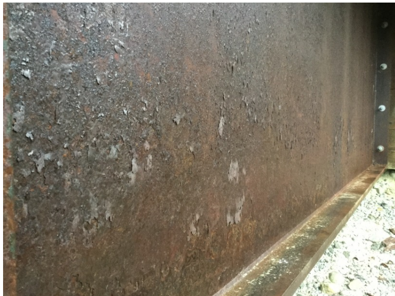
Corrosion on girders
